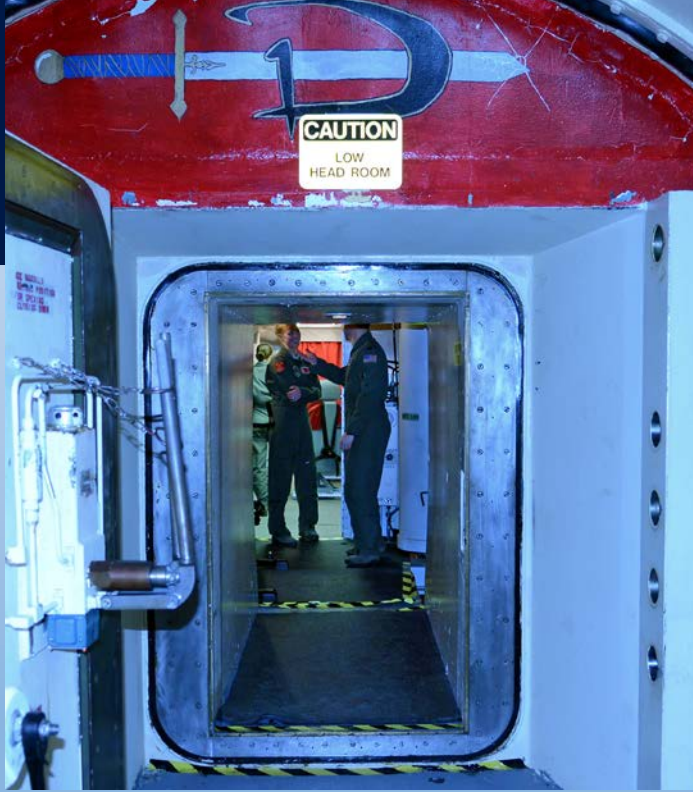
Beyond an eight-ton blast door is a suspended walkway and then the LCC, where missileers pull 24-hour alerts. (Photo: Dan Sagalyn/PBS News Hour)
